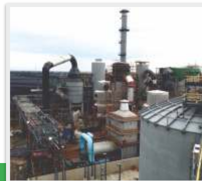
Acid Contact Area In Sulphuric Acid Plant at Mopani Copper Mines, mufulira, Zambia
