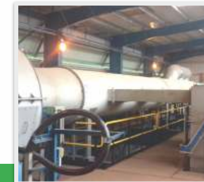
Bag Filter Inter Connecting Duct Assembly For ASFD at Mutanda Mining, Kolwezi, D R Congo
