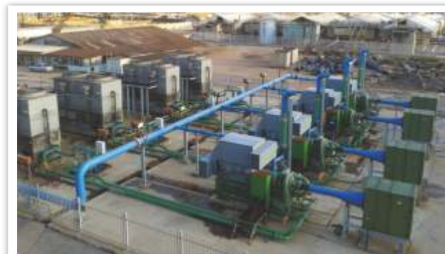
Cooling Towers & Compressors at TLP, Konkola Copper Mines, Zambia
