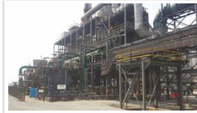
Contact Acid Area at Sulphuric Acid Plant, Mopani Copper Mines, Mufulira, Zambia
