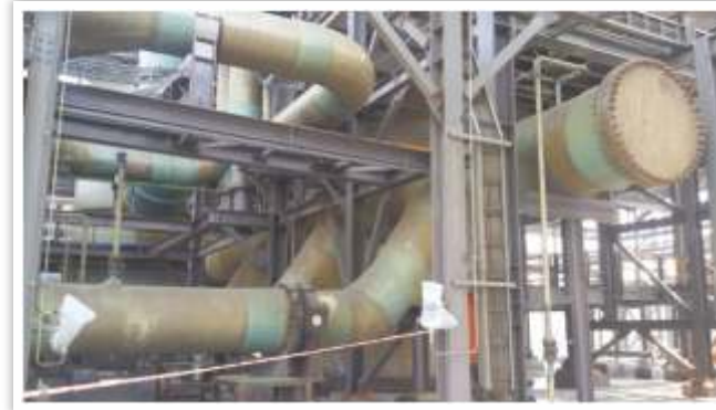
FRP & RTRP Piping at Sulphuric Acid Plant, Mopani Copper Mines, Mufulira, Zambia
