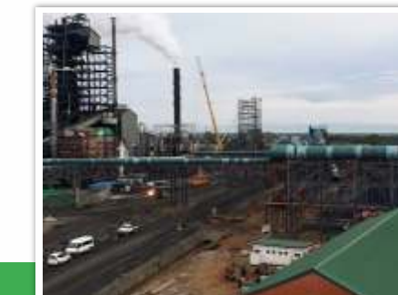
FRP Ducting at Sulphuric Acid Plant, Mopani Copper Mines, Mufulira, Zambia
