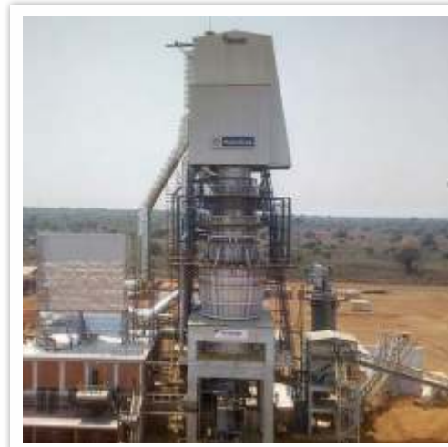
Lime kiln for Handyfa's Lime Plant
