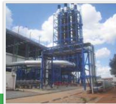
Ducting for Ndola Energy Co. Ltd.
