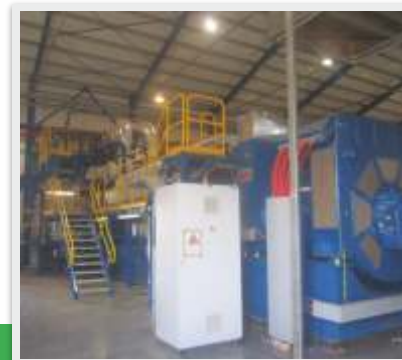
Engine hall for Ndola Energy Co. Ltd.
