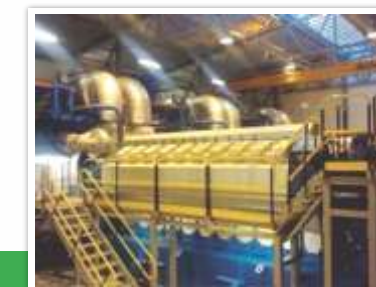
W20V32 Engine generator set for Wartsila project, Zambia
