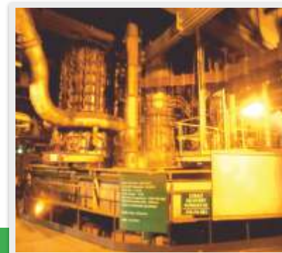
Cobalt Recovery Furnace (CRF) for KCM
