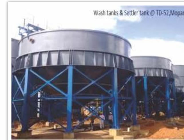
Wash Tanks & Settler Tank @ TD-52, Mopani, Kitwe
