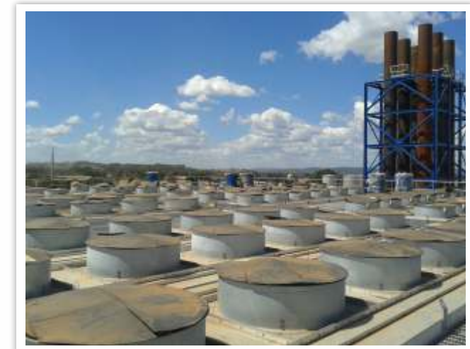
Low Noise Radiators for Engine Hall (50 MW Power Plant @ Ndola Energy, Ndola)
