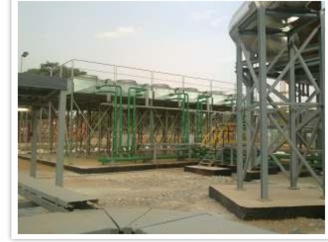
Cooling Tower & its Piping for Wartsila Project, Zambia
