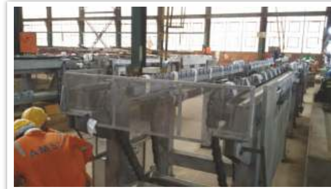
Anode Preparation & Cathode Handling Plant at Mopani Copper Mines, Mufulira, Zambia
