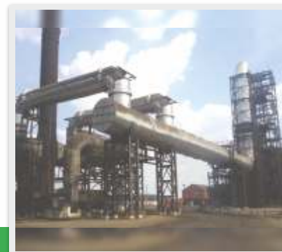
Hot Gas Ducts At Sulphuric Acid Plant, Mopani Copper Mines, Mufulira, Zambia
