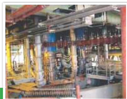
SS & Cu Piping at Smelter
