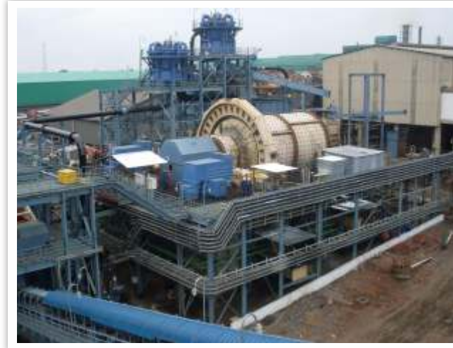
750 TPH Copper Ore Fine Crushing SAG and Ball Mill at Concentrator, Konkola Copper Mines, Zambia
