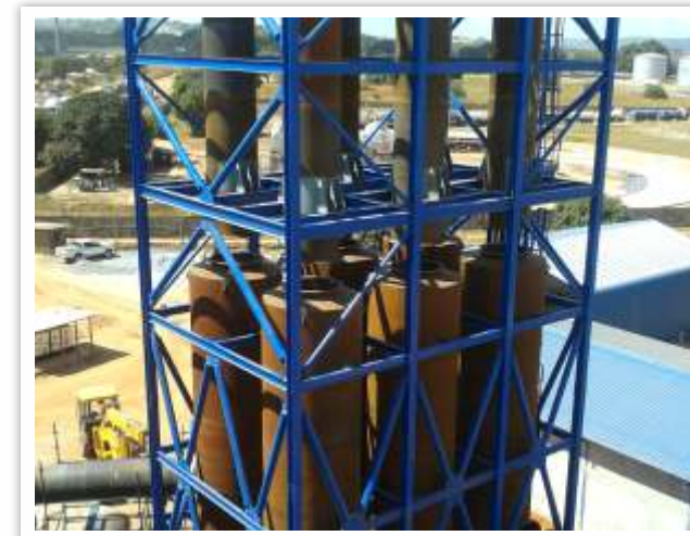
Exhaust Gas Stack for 50 MW Power Plant at Ndola Energy Co Ltd, Zambia
