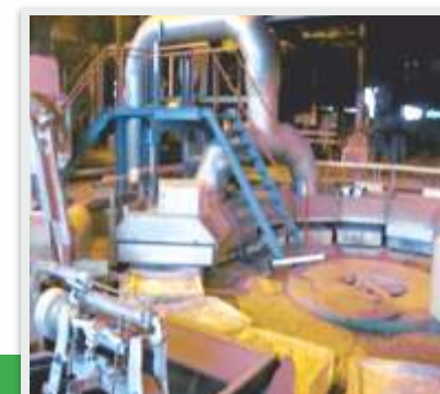
Cast Wheel Exhaust Duct, Nkana, KCM
